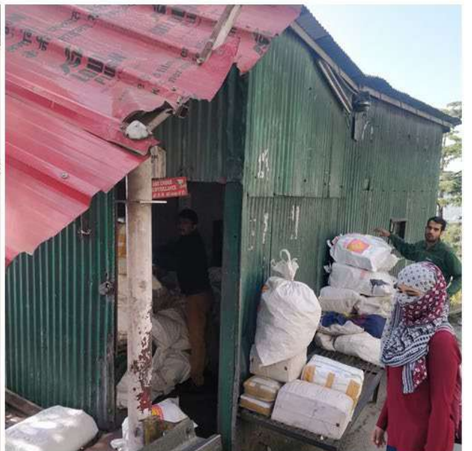
Figure 20: Replacement with incompatible material -- Shimla Railway Station
