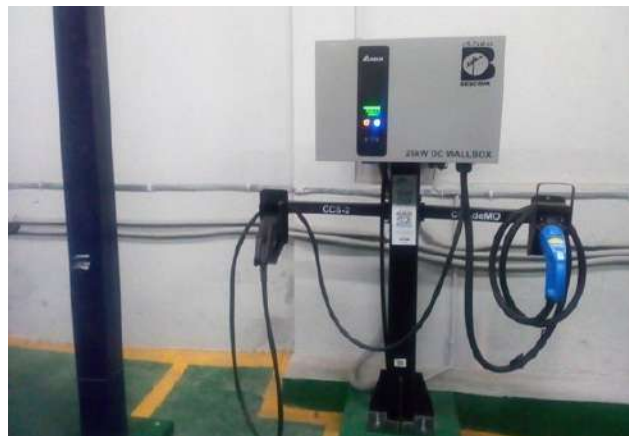
Figure 1-1: Fast DC - CCS/CHAdEMO charger
